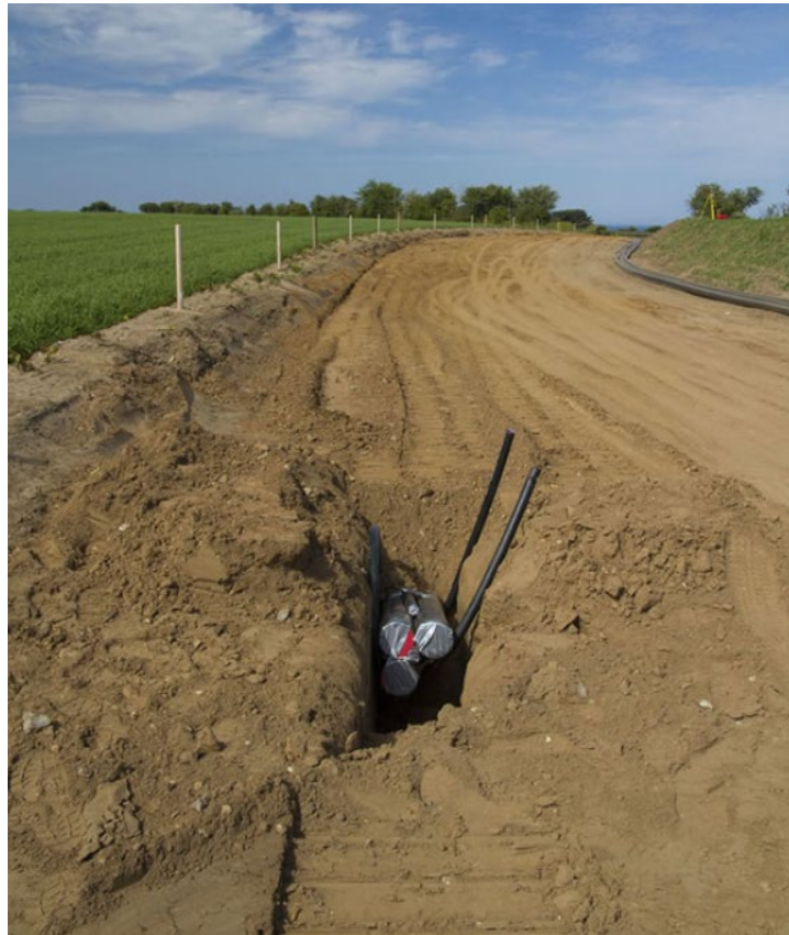
Plate 4-22: Example of backfilled trench following duct installation. End of duct visible in foreground awaiting joint bay construction and cable pulling (Source: Equinor)
